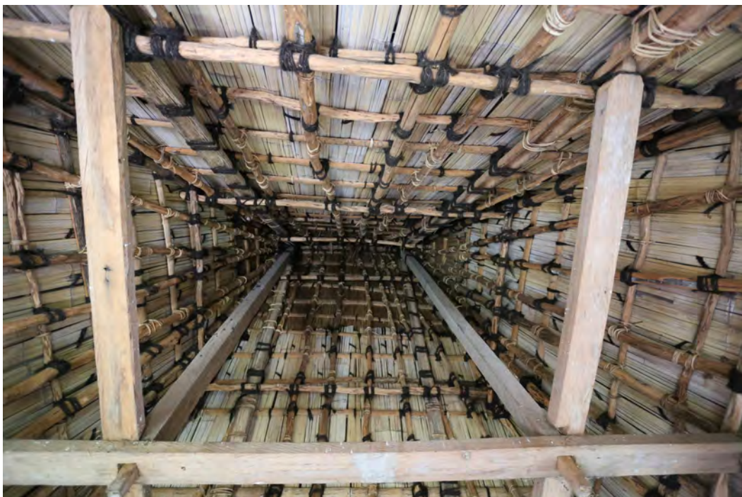
Fig 2. Internal lining of a traditional housing (Uma Lulik) in timber and bamboo in Los Palos
